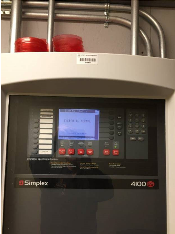
Example 21. Fire Alarm Panel
