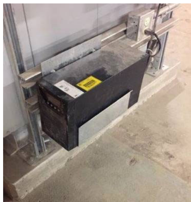
Example 40. Controls UPS
