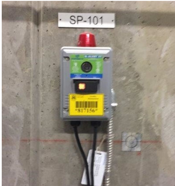
Example 45. Pump Controller
