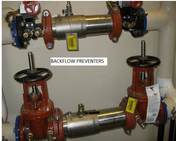
Example 3. Backflow Preventors
