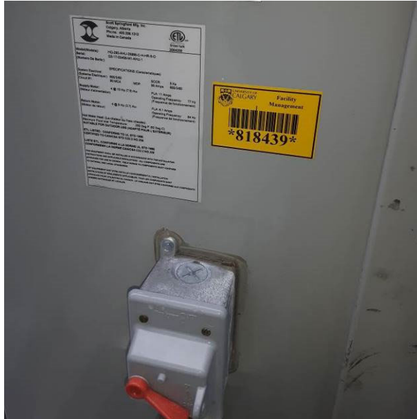
Example 1. Air Handling Unit
