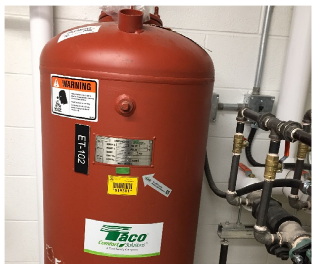
Example 16. Expansion Tank
