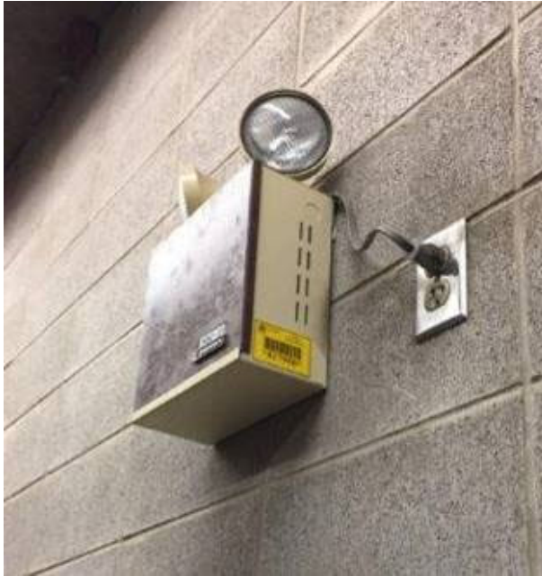
Example 37. Emergency Lighting Battery Pack
