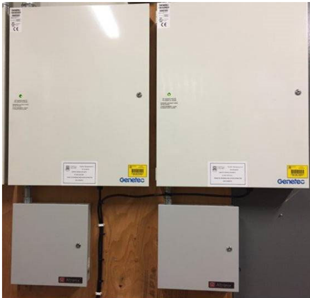
Example 31. Door Access Panels
