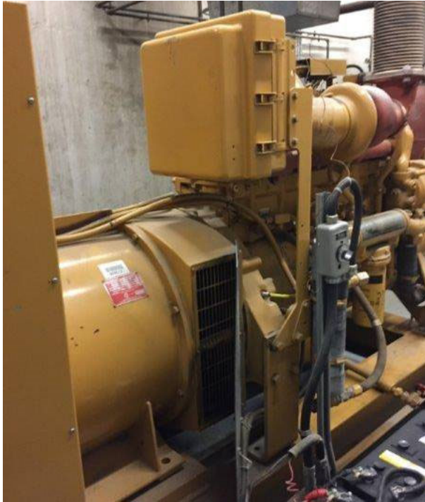
Example 33. Indoor Generator
