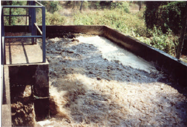
Water treatment plant of CIDADE - De - GOA (A locally owned 5 - star hotel in GOA).
